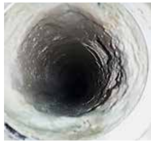
2 weeks after Vulcan was installed, scale had been softer and fallen out.
