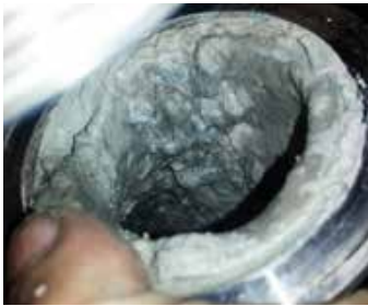
Before Vulcan installation: the pipe was full of scale deposits.
