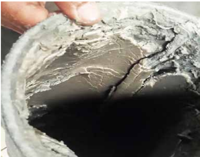
Without Vulcan, the filter was quickly stuck by scale deposits, and it had to be changed every 48 hours.
