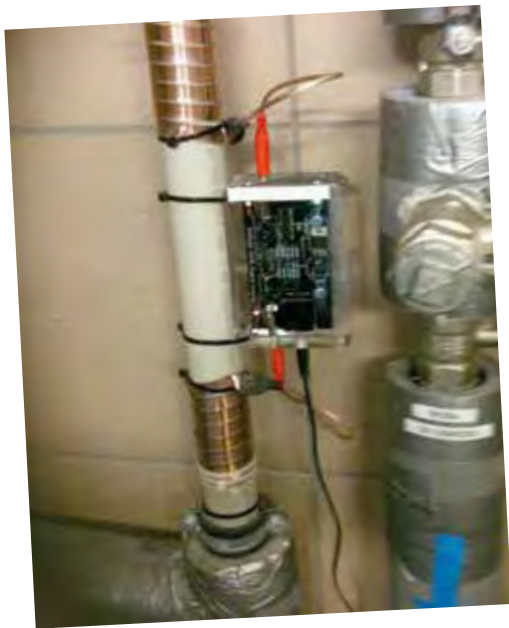
Installation des Vulcan Systems.
