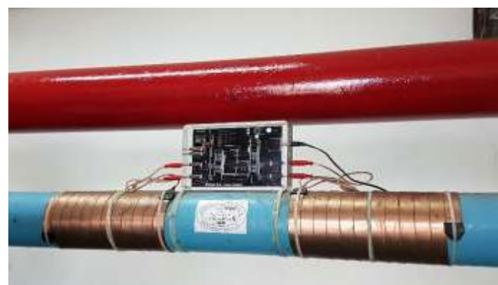
Anti-Scale System Vulcan S25 installed
