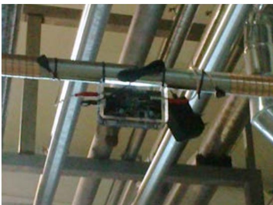
Vulcan 3000 installed in the Delice Danone factory
